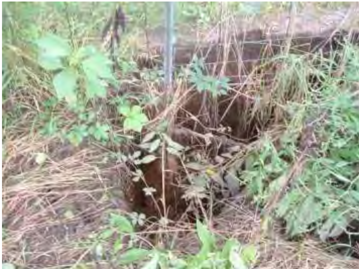
Figure 3.94. Photo of Sinkhole Near Runnells, July 28, 2010
