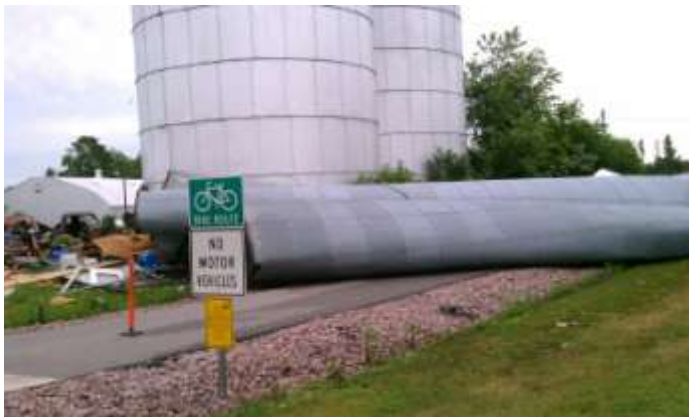
Figure 3.98. Severe Thunderstorm Caused Grain Bin Collapse, July 11, 2011
