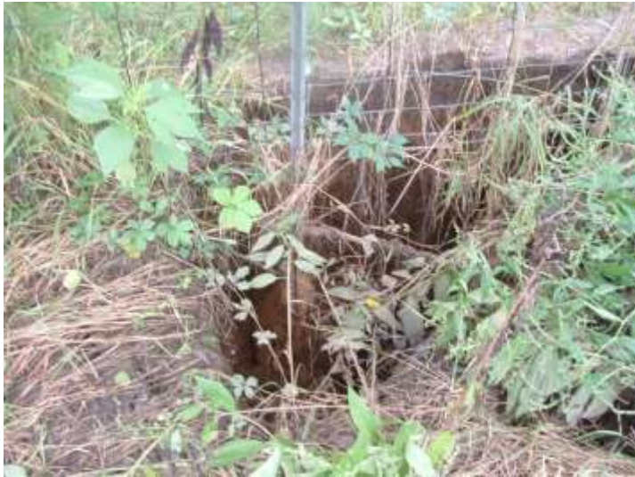
Figure 3.94. Photo of Sinkhole Near Runnells, July 28, 2010
